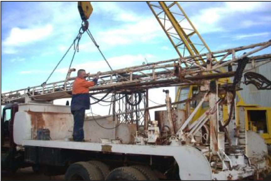
Trevor Orr, UraniumSA Maintenance Manager, unmounting the Mayhew 1000 series drill rig platform and mast from the 6x4 drive White Constructor truck.
