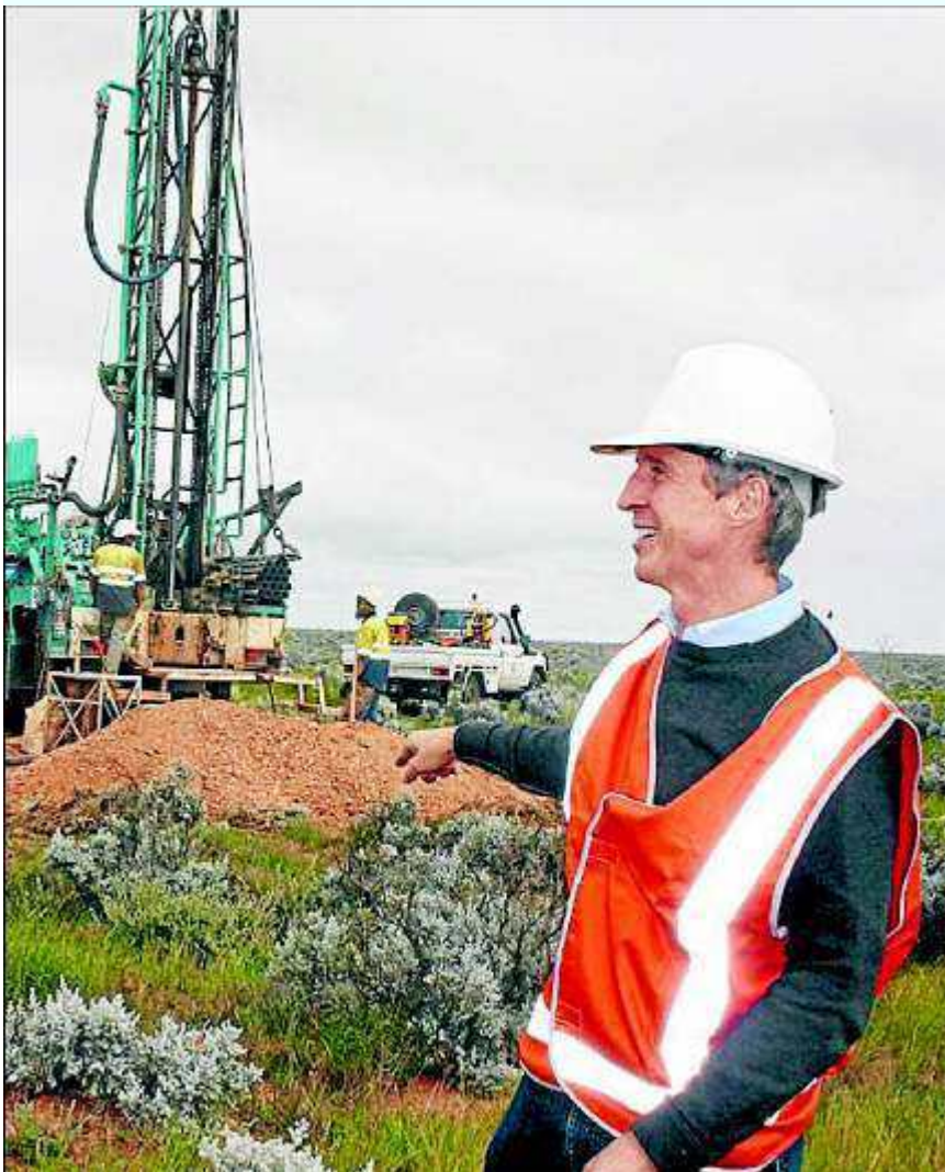
PROGRESSING: General manager for the project Alistair Muir at the site during a visit earlier this year.
