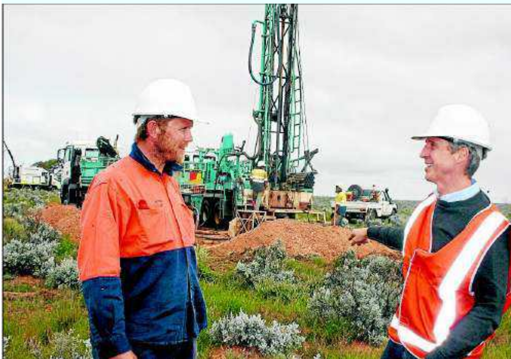
PROGRESSING: Having a chat at the drilling site at Mullaquana were site supervisor Julian Snook (left) and general manager for the project Alistair Muir.
