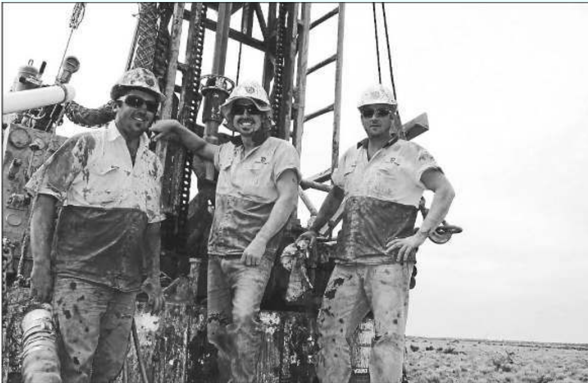
Riggers busy working at the drilling site were: (from left) Christian Cackburn, Jon Scott and Doug Marks of Thompson Drilling.
